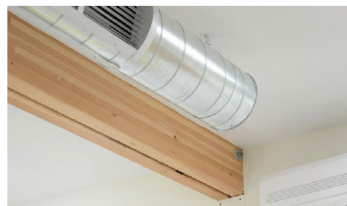
HVAC provides clean, healthy air.
